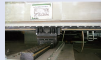
THK products in use at the Disaster Mitigation Research Building; the internal structure can be viewed from the outside.
