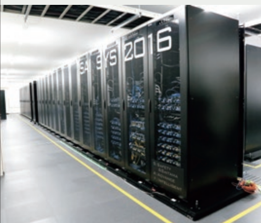
Seismic isolation devices safeguarding our servers
