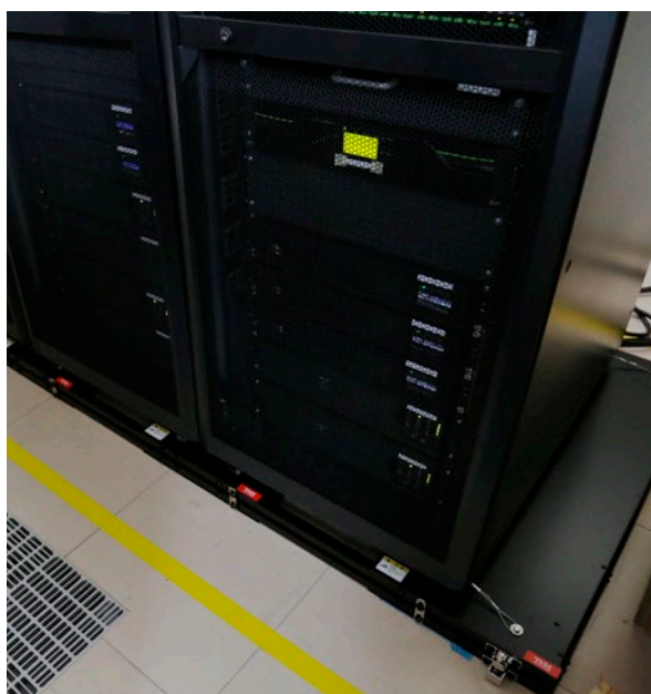
Seismic isolation systems used to prevent the server racks from falling over during an earthquake
