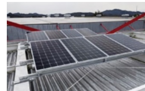
Solar panels (Yamaguchi Plant)
