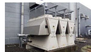
Utilizing small air conditioning equipment (Gifu Plant)
