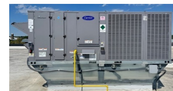
New HVAC unit (TMA)
