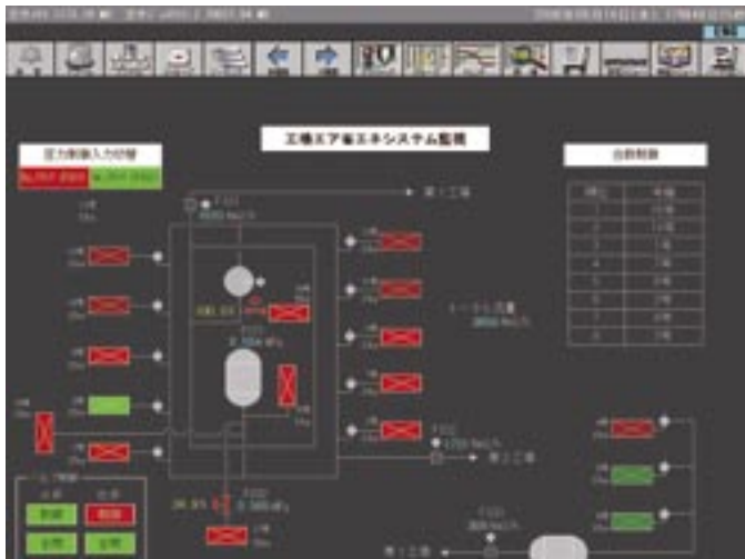
Compressor surveillance monitor screen
