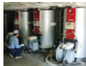
Boiler at the YAMAGUCHI Plant
