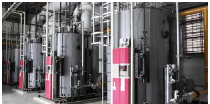
LPG-fired steam boilers
